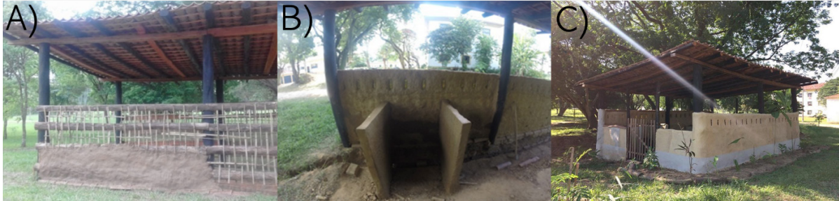
Fig. 1 Construction of the composting patio for the application of Hot Composting Berkeley Method in food waste. Original photos by Bruna Marraccini Precioso de Oliveira and “Composta Rural Group”
