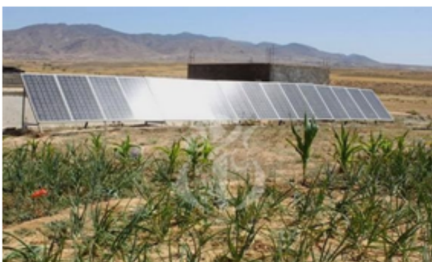
Figure 5. Solar panel solar panel (Algerian region).
