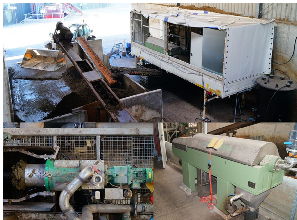
Fig. 2 Installed separation equipment, top: container with decanter centrifuge; left: screw press separator; right: decanter centrifuge
