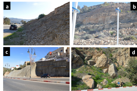
Figure 2. a) Landslide on national road 2. b) Landslide on Corniche Sabadia. c) Retaining walls in the Al-Hoceima entrance. d) Rockfall Netting near to the Al-Hoceima port. © TAHER MORAD 2023.
