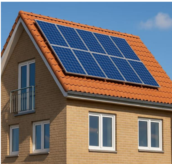
Figure 1. Solar Rooftop PV Panel
